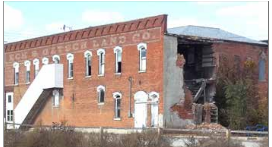
Building on corner, rear caved in – street and sidewalk on south side closed due to danger of falling wall
