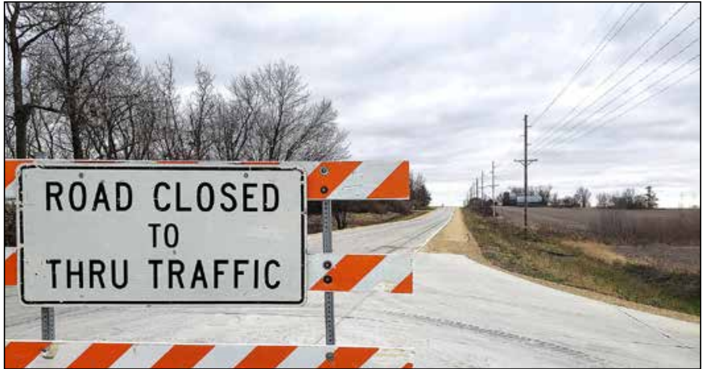
Reed Avenue is finally paved from Highway 3 to C-33. This photo was taken Nov. 14. Photo contributed
